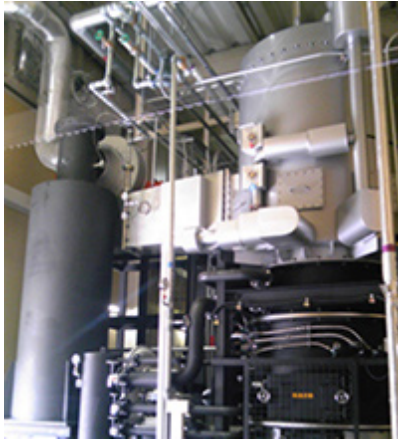
Biomass boiler (Awazu plant)
