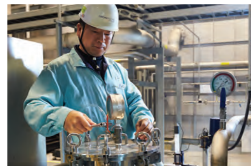
Rainwater Filtering Equipment
