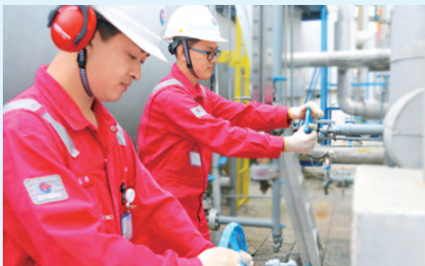
The operator was discharging surplus refrigerant into the newly-added recycling tank.
