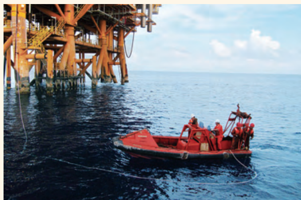
Operating personnel are installing the cabled subsurface buoys for real-time monitoring around the platform.
