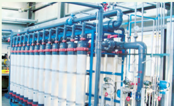
Wastewater Deep Treatment – Reverse Osmosis (RO) Device
