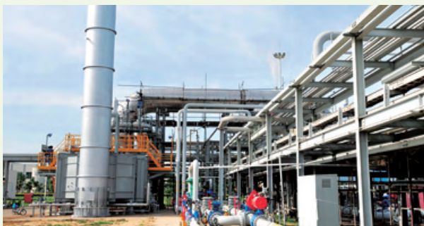
The waste heat recycle unit of Dongfang Terminal Treatment Plant
