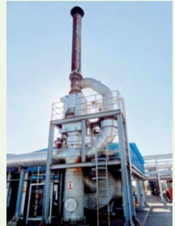
The waste heat recycle unit of thermal medium boiler in Bonan Terminal Treatment Plant Phase I
