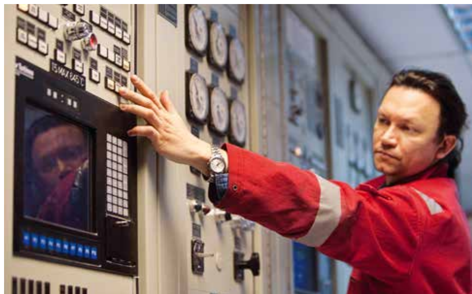
▲ A technician on board our Chirag platform in the Caspian Sea, Azerbaijan.
