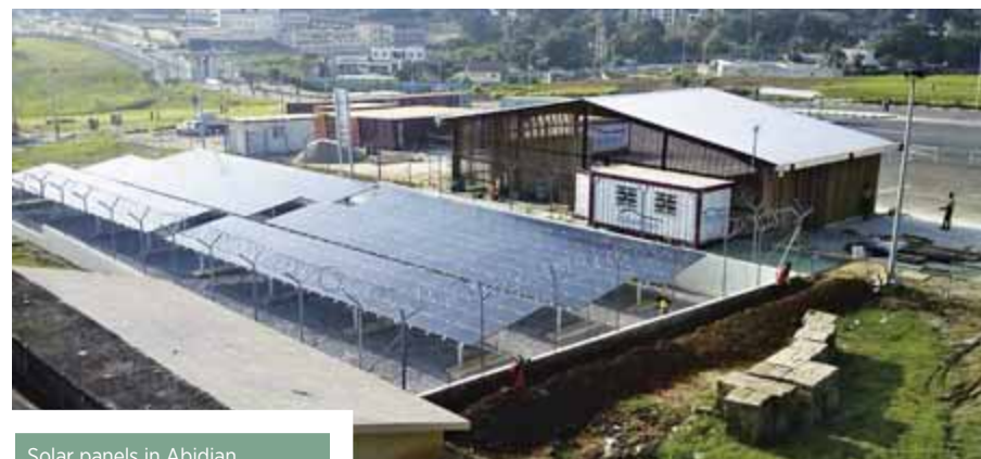
Solar panels in Abidjan.
