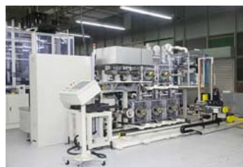
Varnish curing system (protective covers have been removed for this photo)
