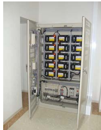
Lithium-ion storage system
