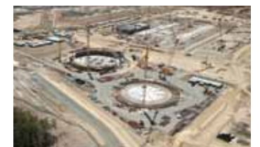
GLNG liquefaction plant in Australia
