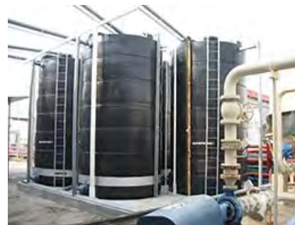
More rainwater tanks (February 2014)
