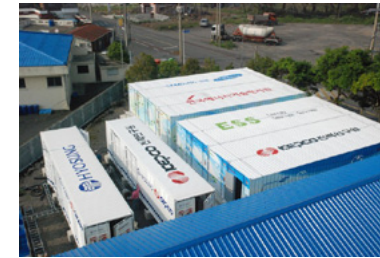
ESS demonstration test site (Jocheon Substation in Jeju)
