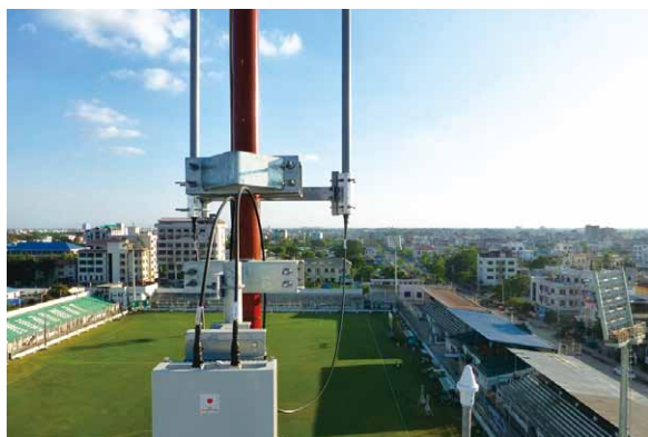
LTE Base Station Installation (Soccer ground in Mandalay, Myanmar)
