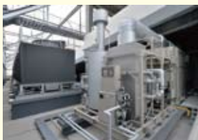
Co-generation systems and long-life emergency generators
