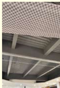
A special construction method with enhanced anti-seismic capability, using an open ceiling design for main walkways to prevent falling objects
