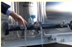
Installation of water tanks (with 380-ton effective capacity) to ensure emergency drinking water supply
