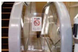
Safety Measures for Escalators
