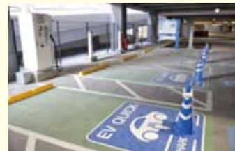
14 electric charger vehicle (EV) station units
