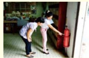
Pointing out the need for a fire extinguisher during a manufacturing plant work environment check.
