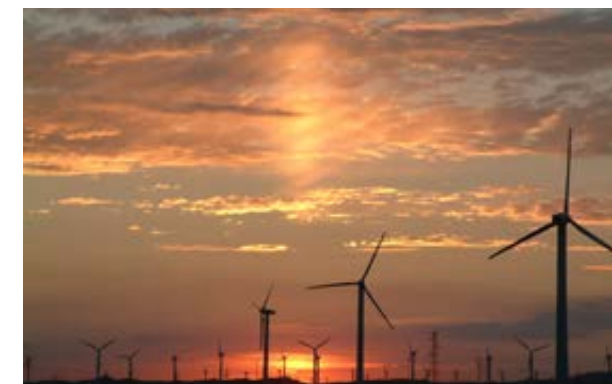
甘肃大唐玉门昌马风电场 Datang Wind Farm in Changma, Yunnan, Gansu Province
