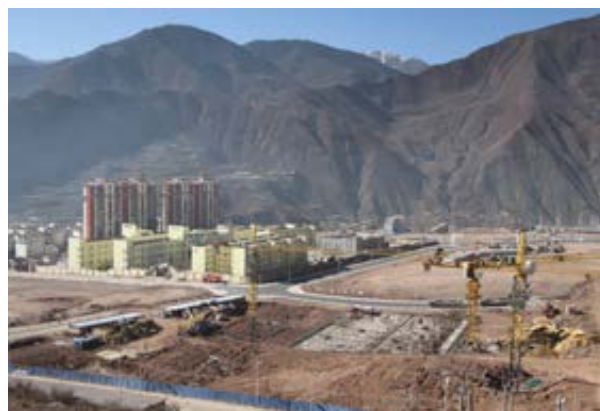
西藏昌都地区公租房项目建设现场 Construction site of public rental housing project in Qamdo, Tibet
