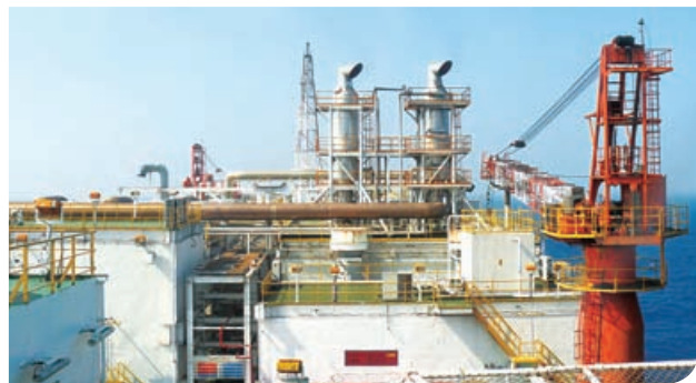
Flue gas utilization devices of FPSO in Panyu Oilfield
