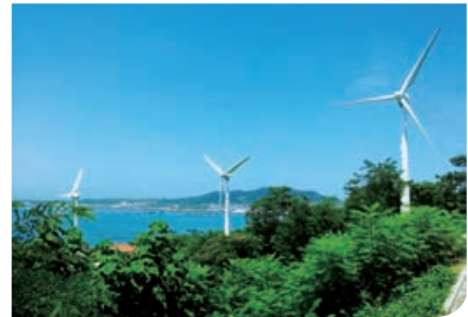
Seashore wind turbine generator
