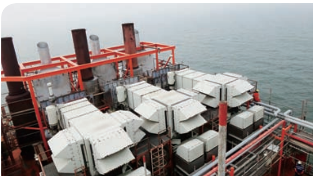
Recovery devices of turbine waste heat in Jinzhou 9-3 Oilfield
