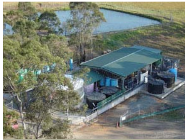
The water filtration plant at our Illawarra Coal Appin West site.
