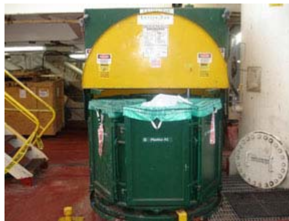
A Six Category Waste Compactor on one of our offshore platforms.
