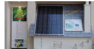
Solar cells for installation on buildings and educational material on solar power displayed in the reception area
