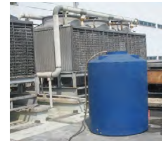
Reducing the factory's environmental impact by installing water recycling equipment on the cooling tower
