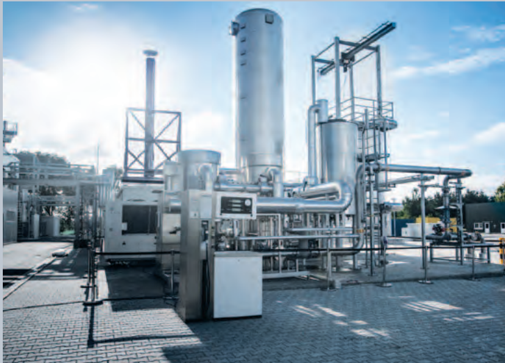
The newly opened Audi e-gas plant in Werlte – built around an MAN methanation reactor. © Audi AG
