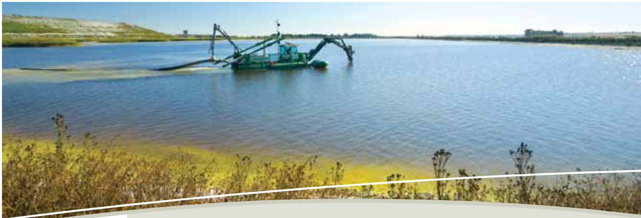
A dredger removing sediment from an evaporator dam to increase capacity for water received from Secunda plants, as well as rain water.
