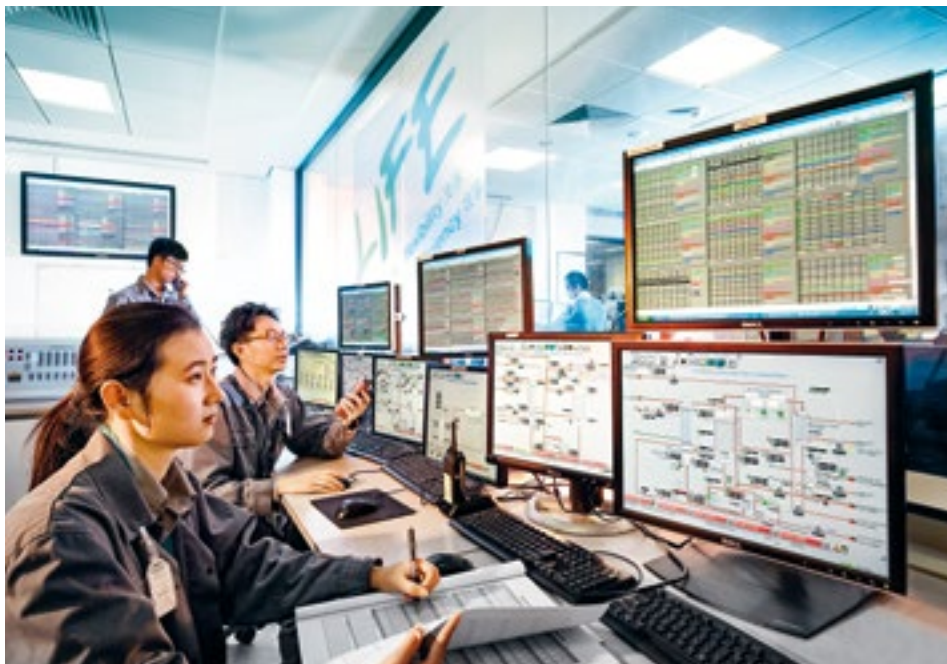
The control room at the MDI plant in Caojing, Shanghai: Bayer employees Fanny Fan (front), Todd Huang (center) and Qi Wu use the STRUCTese™ management system to reduce the facility's energy consumption.
