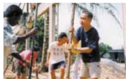
Aviva staff help build the multi-purpose hall for the Orang Asli community in Malaysia.
