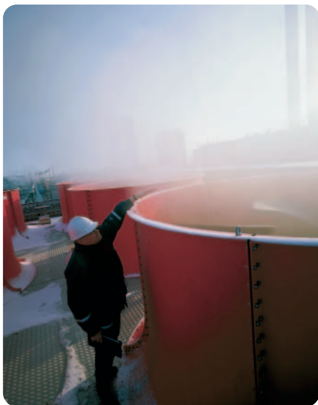
Cooling towers in Kalundborg. Most of the consumption of energy and the CO 2 emissions relate to supply plants, eg air compressors, pumps, ventilation and cooling, for our production processes. These areas are therefore highlighted in Novo Nordisk's CO 2 strategy.
