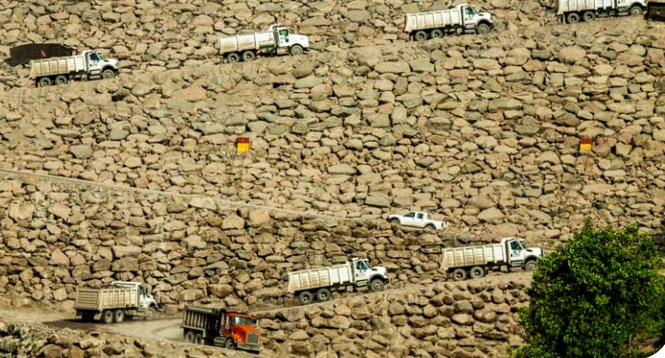
Transport at the Sogamoso Hydroelectric Power Plant
