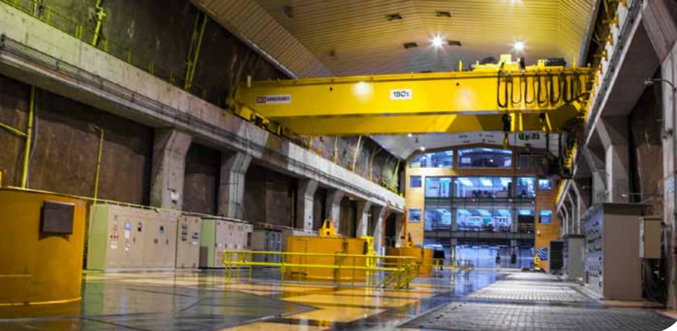
Jaguas Hydroelectric Power Plant
