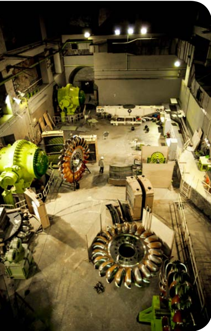
San Carlos Hydroelectric Power Plant
