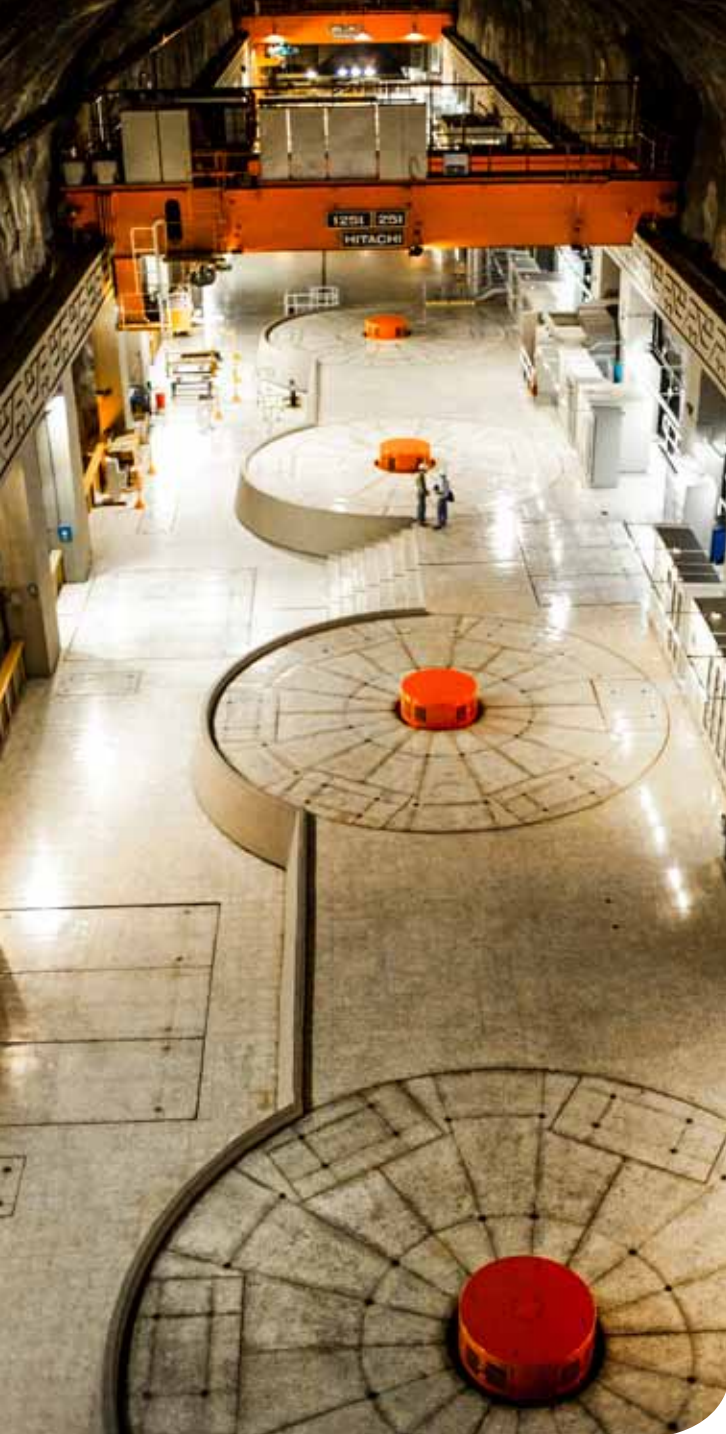
San Carlos Hydroelectric Power Plant
