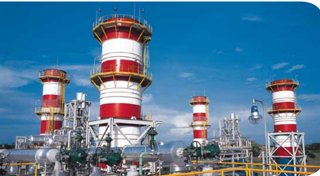
Termocentro Power Plant
