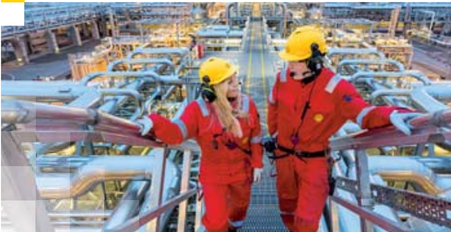
Shell employees working at the Ormen Lange gas processing plant, Norway.
