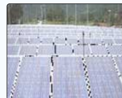
▶New solar energy module panels
