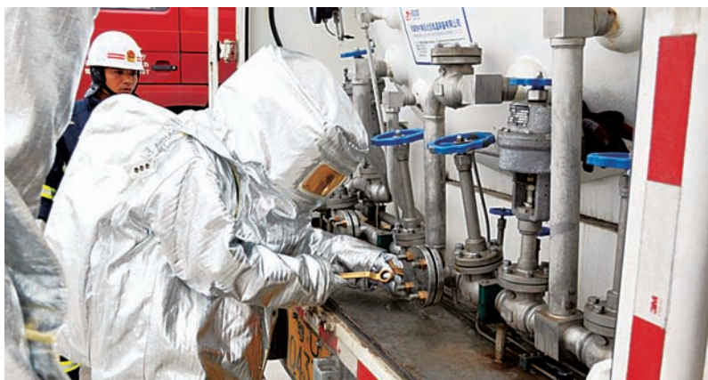
An emergency repair personnel wearing a respirator and fire proximity suit, is working on closing a valve on the LNG tank car
