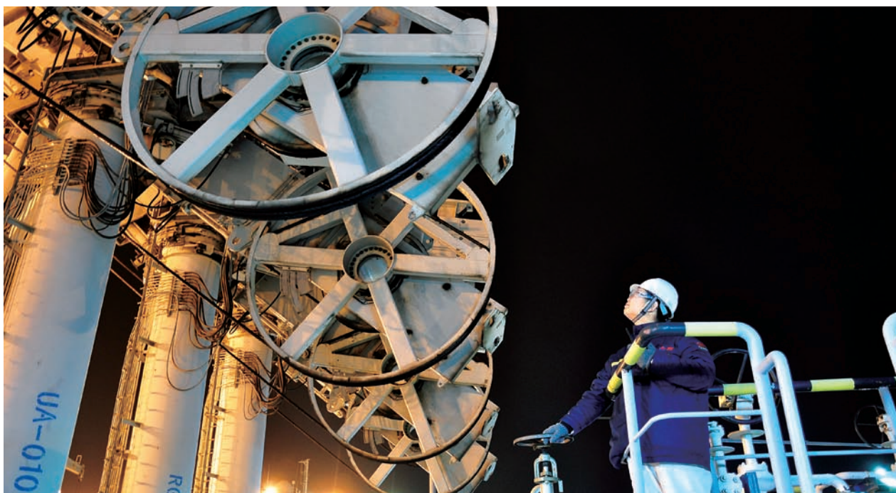
An employee on duty in Fujian putting extra effort during an inspection tour to ensure adequate LNG supplies for winter
