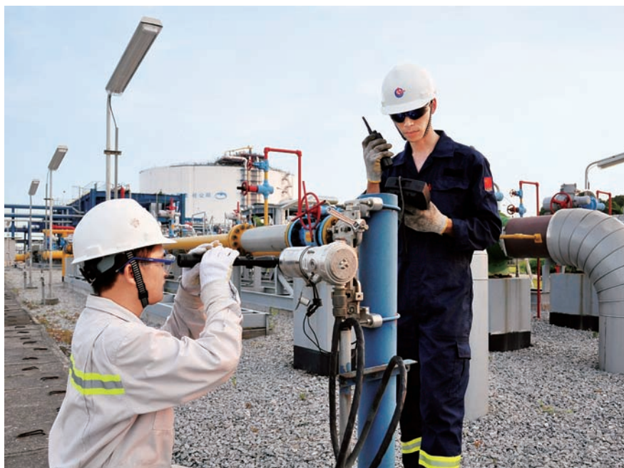
Engineers conducting inspection and maintenance of fire and gas equipment at an LNG station pipeline facility
