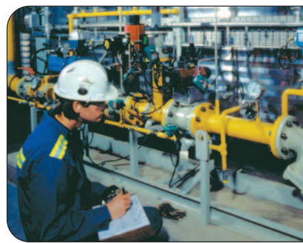
Talisman completed construction of a 10-megawatt cogeneration power plant in Edson, Alberta, in 2004.
