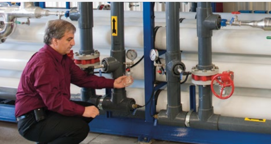
Water reclamation system at Frito-Lay plant.
