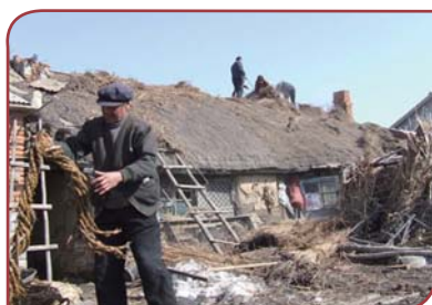
泥草房改造前 Before renovation
