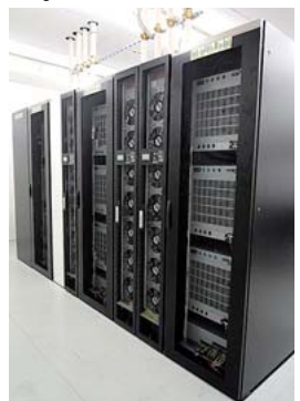
Modular data center
