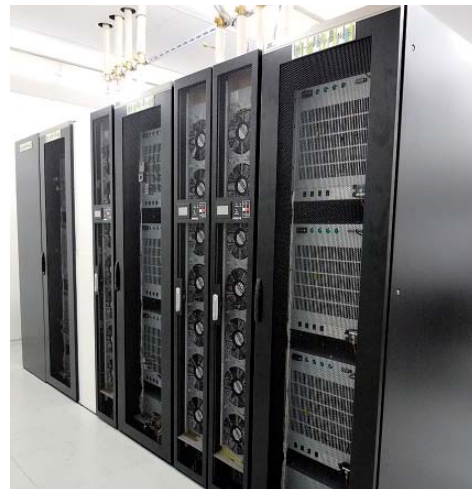
Modular data center
