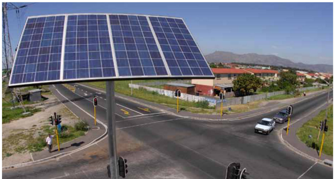
A demonstration solar-powered traffic light in the Western Cape.
