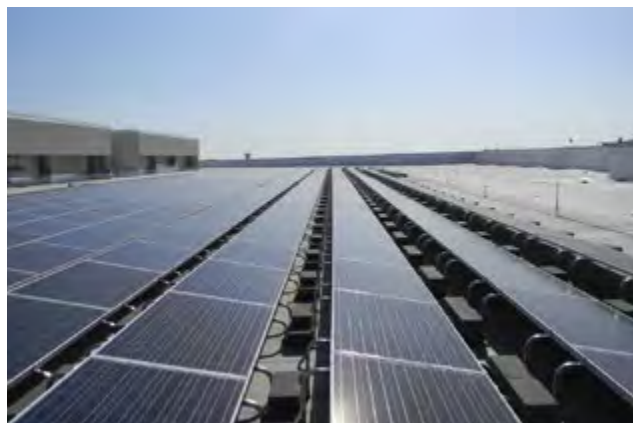
Solar array at Cisco's Allen, Texas data center
