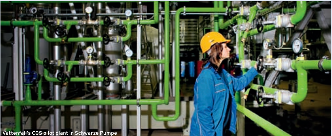
Vattenfall's CCS pilot plant in Schwarze Pumpe
