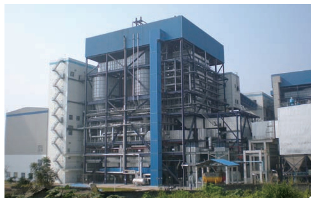
First home made 330 MW circulating fluidized bed boiler developed by Xi'an Thermal Power Research Institute Co.,Ltd.
