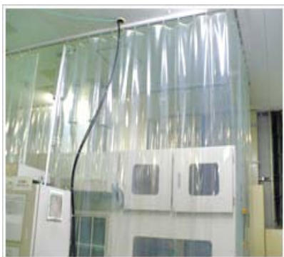
Countermeasure to exhaust heat from large drying furnace
