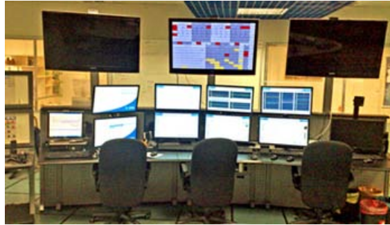
Central control room
