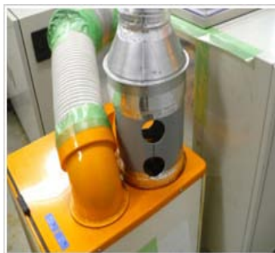
Countermeasure to exhaust heat from spot cooler
