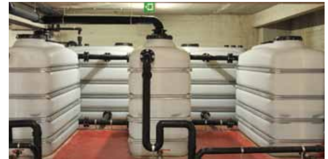
Top: Accenture's flex-fuel cars and recycling facilities in Brazil. Bottom: Accenture rain-water collection facility in Brussels.
