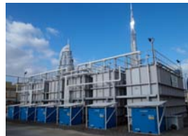
Wastewater recycling plant (Dubai, UAE)*
