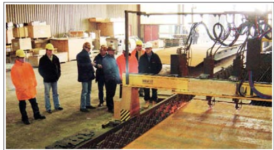
Steel plates for the De Ruyter project are cut at Zwijndrecht in the Netherlands. Suppliers were selected not only for their competitiveness, but also for their health, safety and environmental track records.
