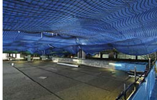
The innovative scaffolding used to protect employees during works at Salmesbury, England.
