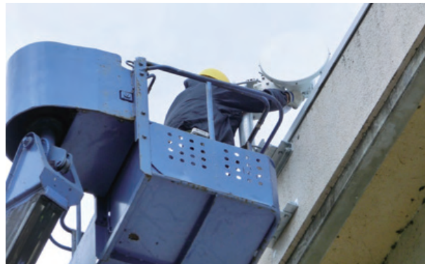
Network equipment is installed on an elementary school building
