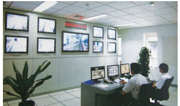
The wireless system control room of the Huichen Senior Service Group
