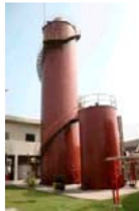
Wastewater Treatment Plant at AmBev's Huachipa, Plant near Lima, Peru.
