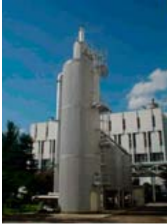
Heat recovery and hot water tank at Icheon plant, Korea.
