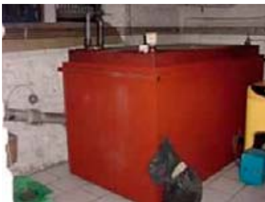
An upgraded fuel storage installation in a private house in the Jupille community in Belgium.
