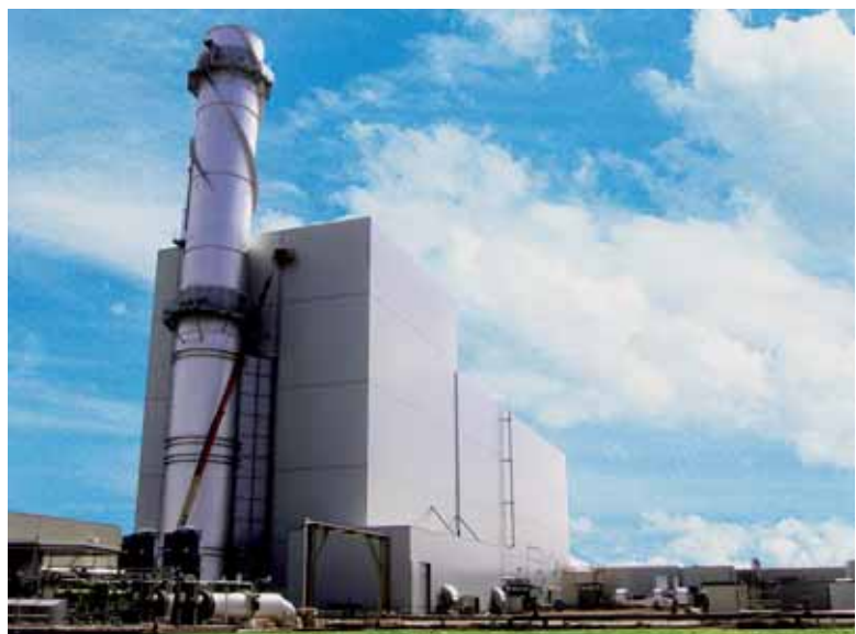
The Castejón combined cycle power plant (Navarra) holds the EMAS distinction.
