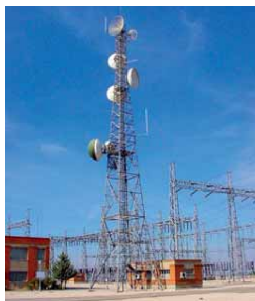
View of a substation and its communications infrastructure.
