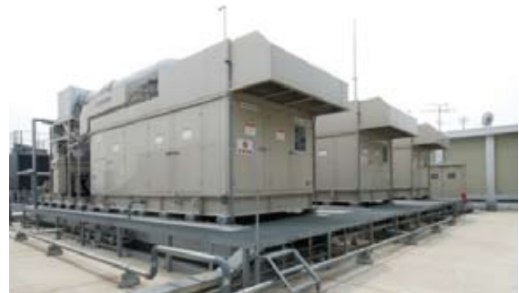
Private power generation equipment installation
