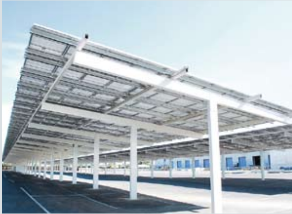
The solar energy system at our location in Sacramento.
