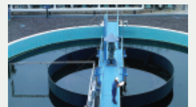
Wastewater Treatment Plant
