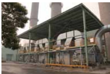
Baosteel Co., Ltd. 1880 Hot Rolling Production Line Reheating Furnace Waste Heat Recovery Project
