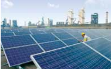
Energy Centre Building 130 KW Photovoltaic System Project
