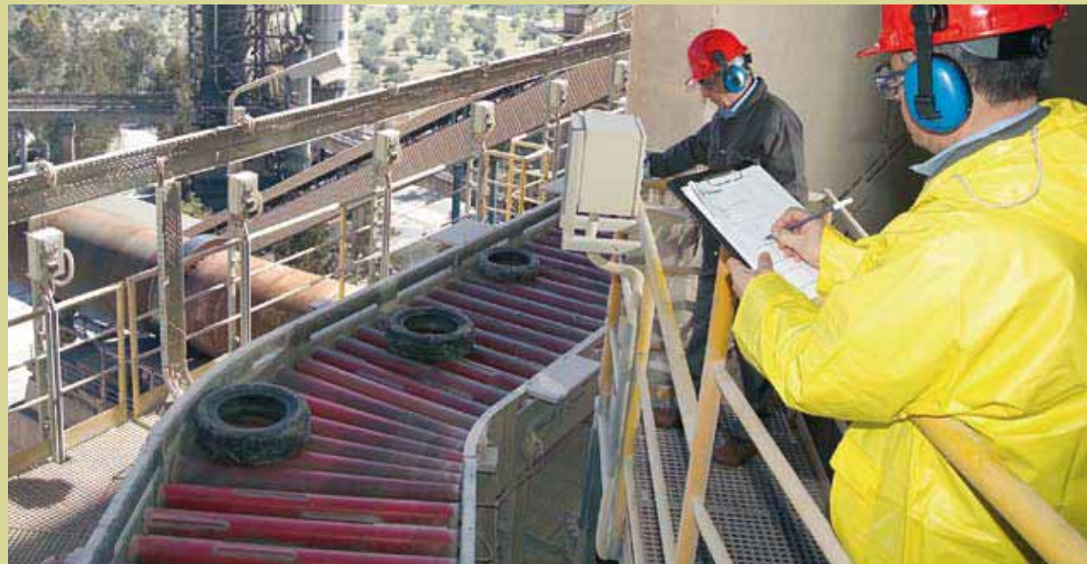
New feeding line for tires, Kamari plant, Greece, 2006
