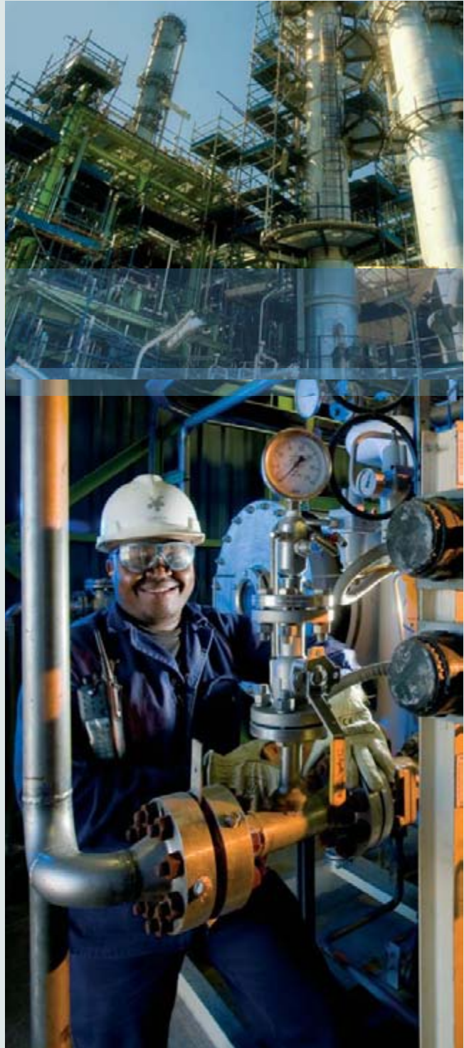
Pule Letuba, process controller at the Secunda water recycling project, checks an ozone generator unit.
