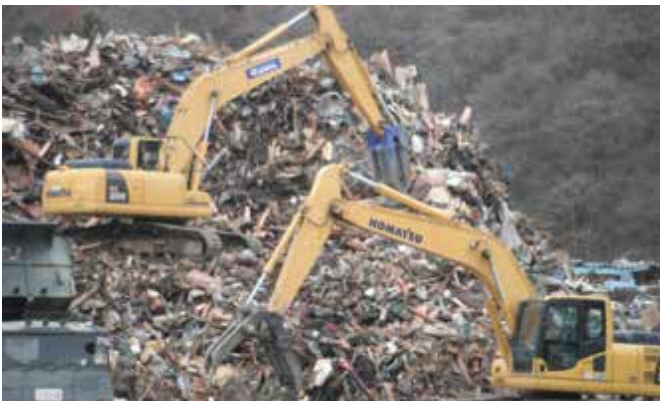
●● Hydraulic excavator in operation in Onagawa, Miyagi Prefecture, where removal of debris was a pressing need
