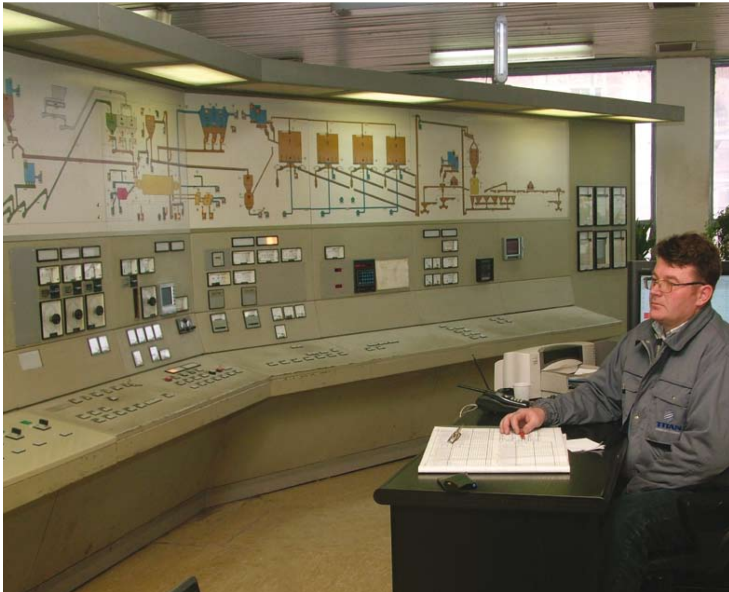
Control centre, Kosjeric plant - Serbia, 2005
