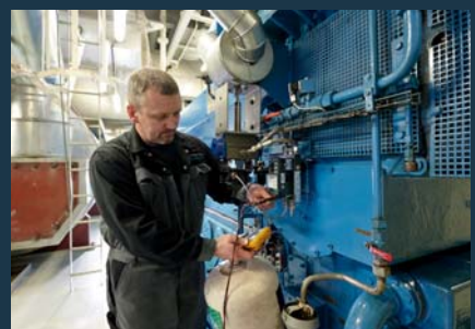
During the test phase, Per Lunde monitors the performance of the SCR system, which was retrofitted to the ferry.
