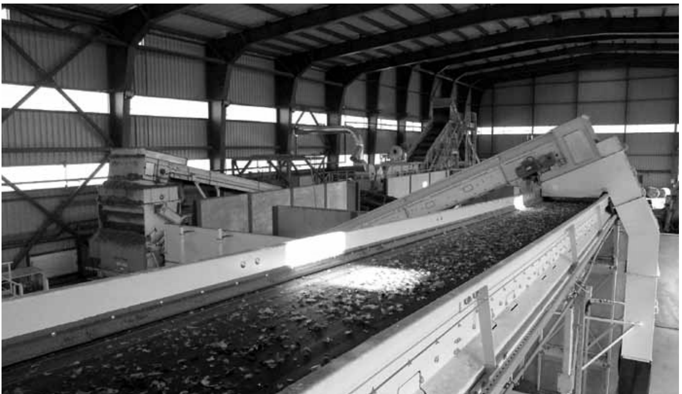
Alternative fuels installation, GAEA Bulgaria
